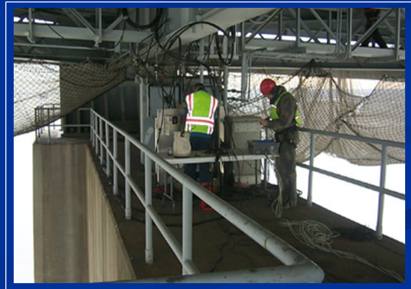
Preparation of the Pier Cabinet for DAQ
